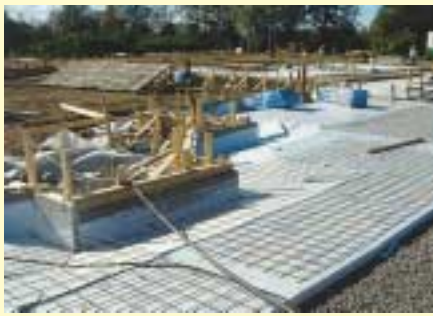
Left, concrete/eps slab-edge insulated forms and sub-slab insulation on FPSF for an elementary school in Stockholm, Sweden. In Norway, Sweden and Finland, 2-inch thick sub-slab insulation, either EPS or XPS, is widely used under concrete slabs to keep the concrete warm for thermal comfort. BPA Construction.
