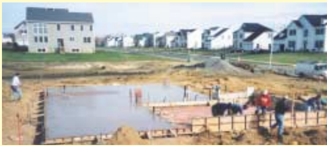
HUD/PATH demonstration house under construction by K. Hovnanian Homes in New Jersey.
