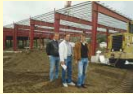
Left, shopping mall in Trondheim, Norway. Steel columns and non-load-bearing walls on FPSFs. A.S. Anlegg Construction. In Scandinavia, reinforced FPSF slabs have been used on other commercial buildings to span weak soil between deep piles.
